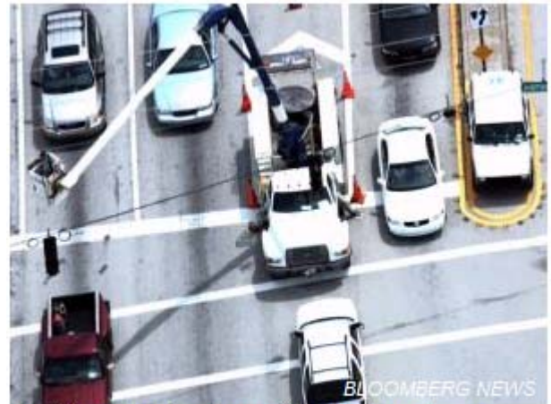
A utility worker in a cherry-picker truck works on a traffic signal in Florida. Photo enforcement is a 'battleground' in the US. Photographer: Bloomberg News.
